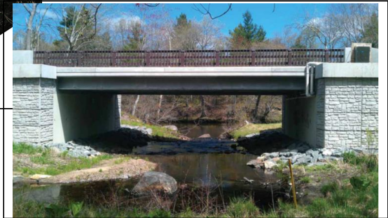
Example of a clear-span bridge which retains the existing river channel, abutments are set back from the river bank (AT&F, 2022)
